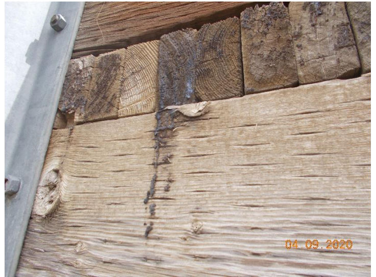
Suspect asbestos-containing material O-19-D-TR01. The tar material is non-detect for asbestos.
